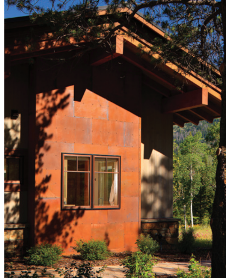
Strout Architects describes the naturally occurring rusty red patina as having a life of its own, one meant to deepen with time as it turns a beautiful rusted red.
